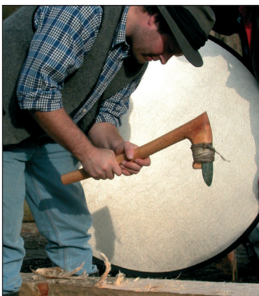
■ Fig. 5 We used an adze shafted on a "kneewood" to flatten the surface of the rectangular posts.
